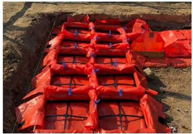
2) Set the formwork.-Open the top surface for filling works. Fill fillings up to the specific volume, then level its surface.
