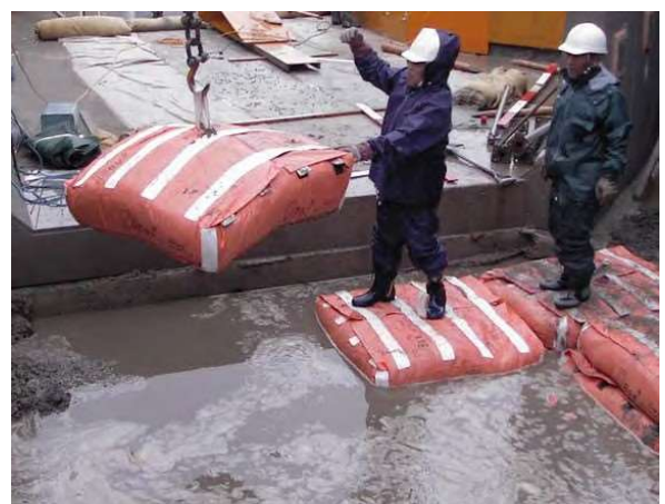
6) An example of a ground reinforcement work of the retaining wall behind the river where the ground has been boiling.
